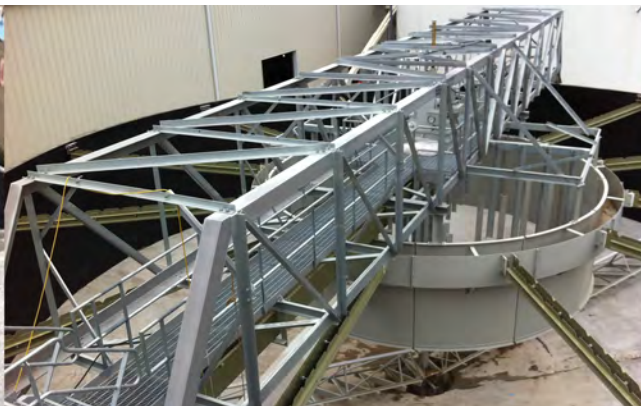
Consol Energy - 80' Diameter Flocculating Clarifier
